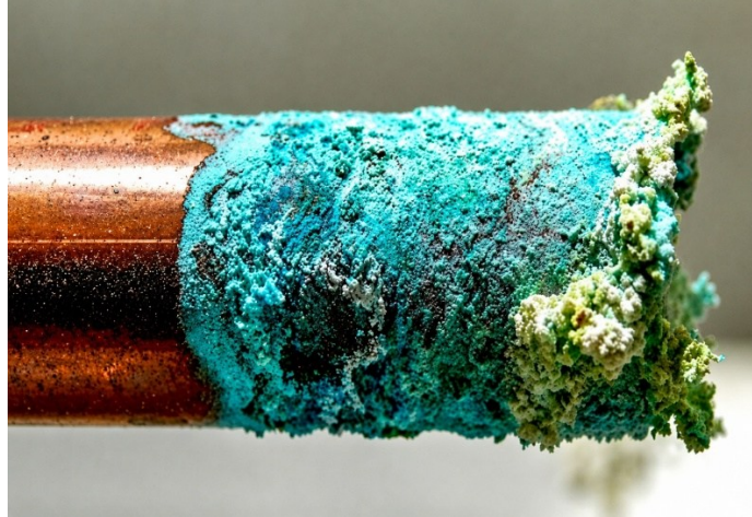
Figure 5. Corrosion and discoloration at aluminum–copper DCU 2 joints were observed on-site.
